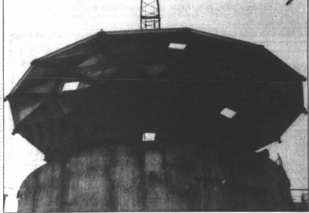
REFINERY UMBRELLA —An aluminum geodesic dome being lowered into place will protect the top of a floating roof tank at Exxon Company's Baton Rouge Refinery. Like and umbrella, the dome will block sun and rain, extending the usable life of the floating roof and minimizing maintenance costs. Skylights will allow operators to monitor the tank for proper operation. The geodesic design lowers installation costs by eliminating the need for internal supports. (AP Laserphoto)
