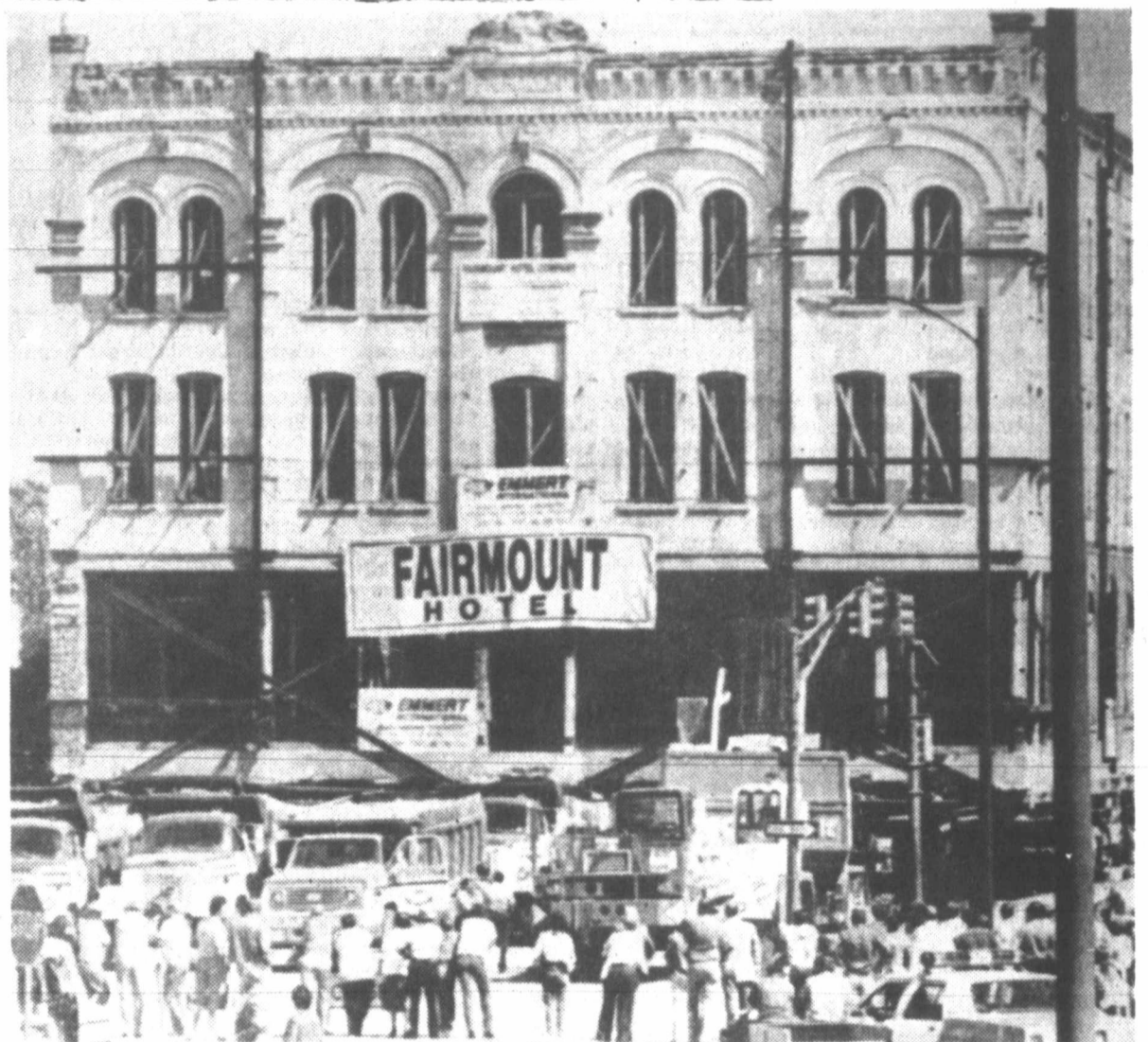
HOTEL MOVE—The Fairmount Hotel, a 79-year-old building weighing 3.2 million pounds, inches its way down Bowie Street in San Antonio Sunday during a four-block move across downtown. The building is to be renovated at its new site. (AP Laserphoto)
