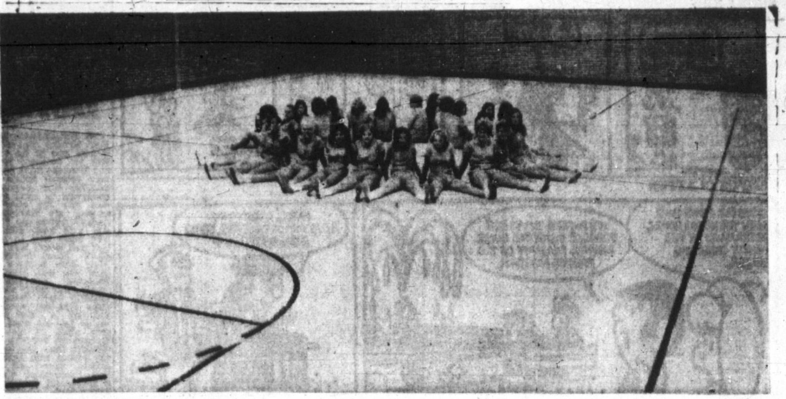
CAMDURA SEAMLESS FLOORS can take the hard wear and tear of gym floors. Pampa High School girls' physical education classes, as well as social and civic functions are conducted on the new Camdura Seamless Floor. Normal traffic in the home will never be called upon to withstand the wear and tear of floors in public buildings, proving that this is the type of long-lasting flooring homeowners should choose. (Staff Photo)
