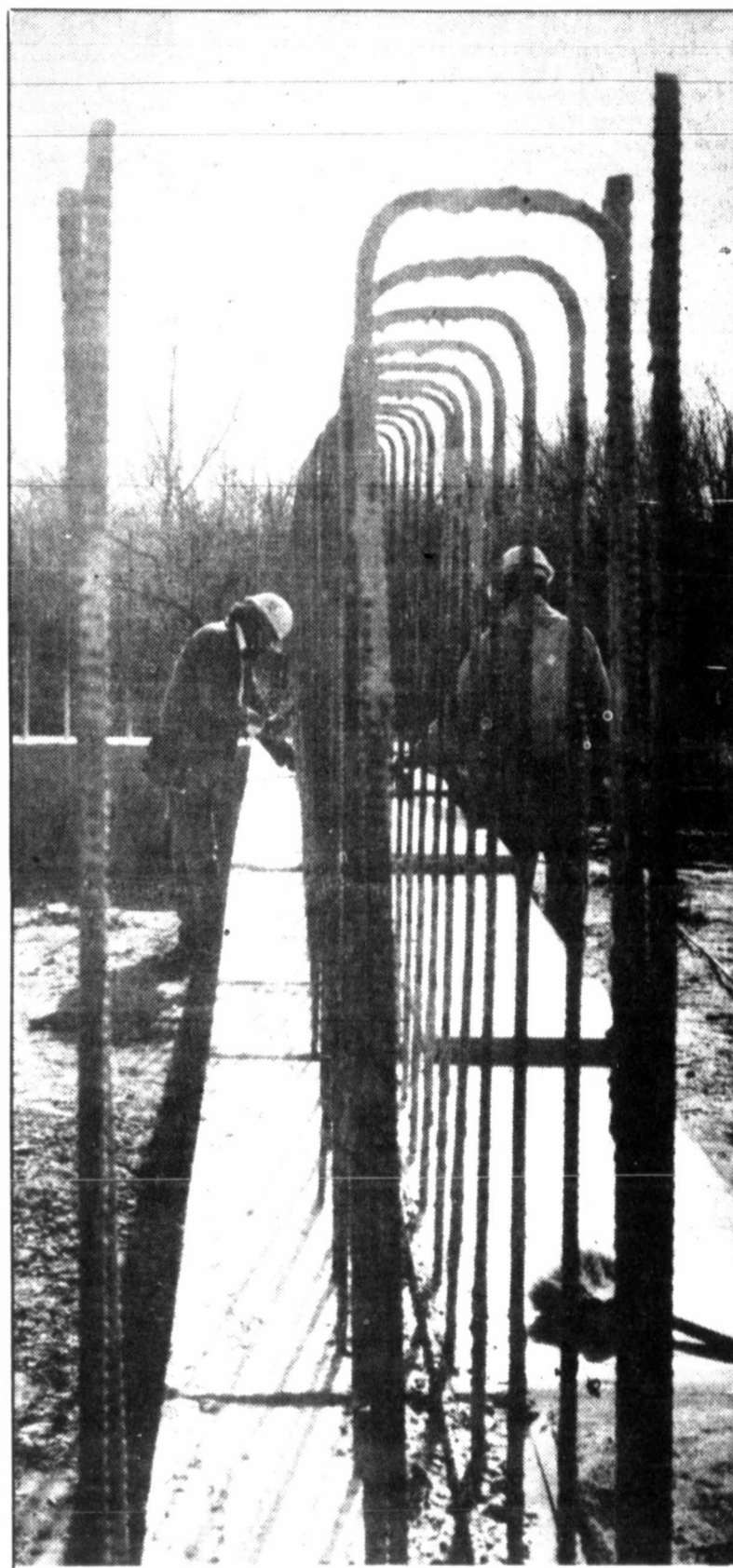
A TALL ORDER — Surrounded by steel support rods, Texas Highway Department workers Joe Segovia (left) and Imon Pennington assemble a support beam for a new bridge on FM 2375 west of Lefors. The new bridge will be 600 feet long and 34 feet wide and is expected to be completed in May. (Photo by Cathy Spaulding)
