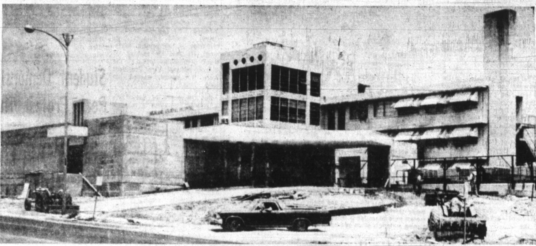
HALFWAY COMPLETED, construction project at Highland General Hospital will add nearly $1.5 million in new medical facilities for the area. The project began last August and is scheduled for completion Nov. 25. Added to present facilities will be a new laboratory, and numerous other medical care facilities, according to a hospital spokesman. (Staff Photo)
