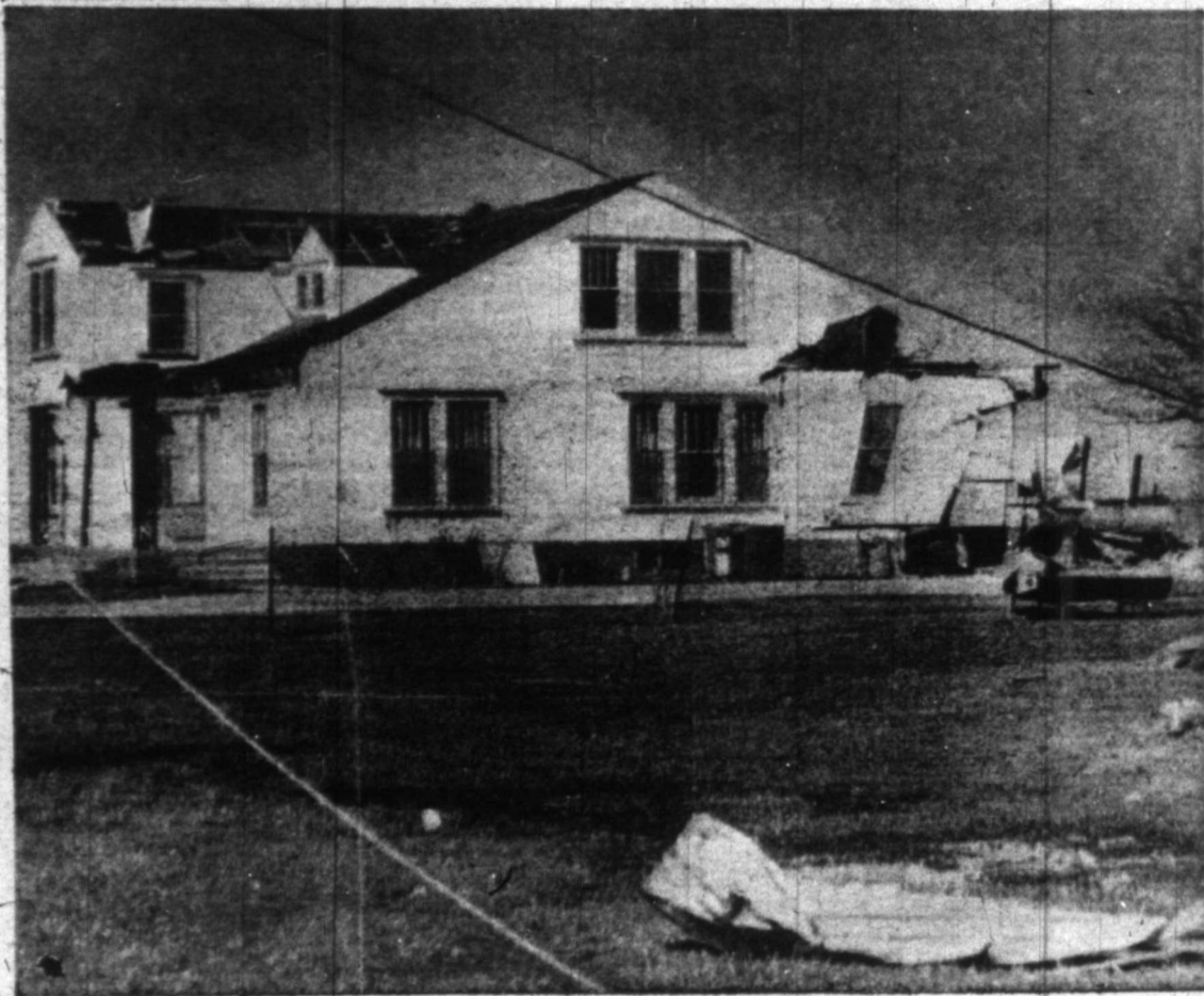
ALL THAT remains of the Charles Williams home located one mile north of McLean on SH 273.
