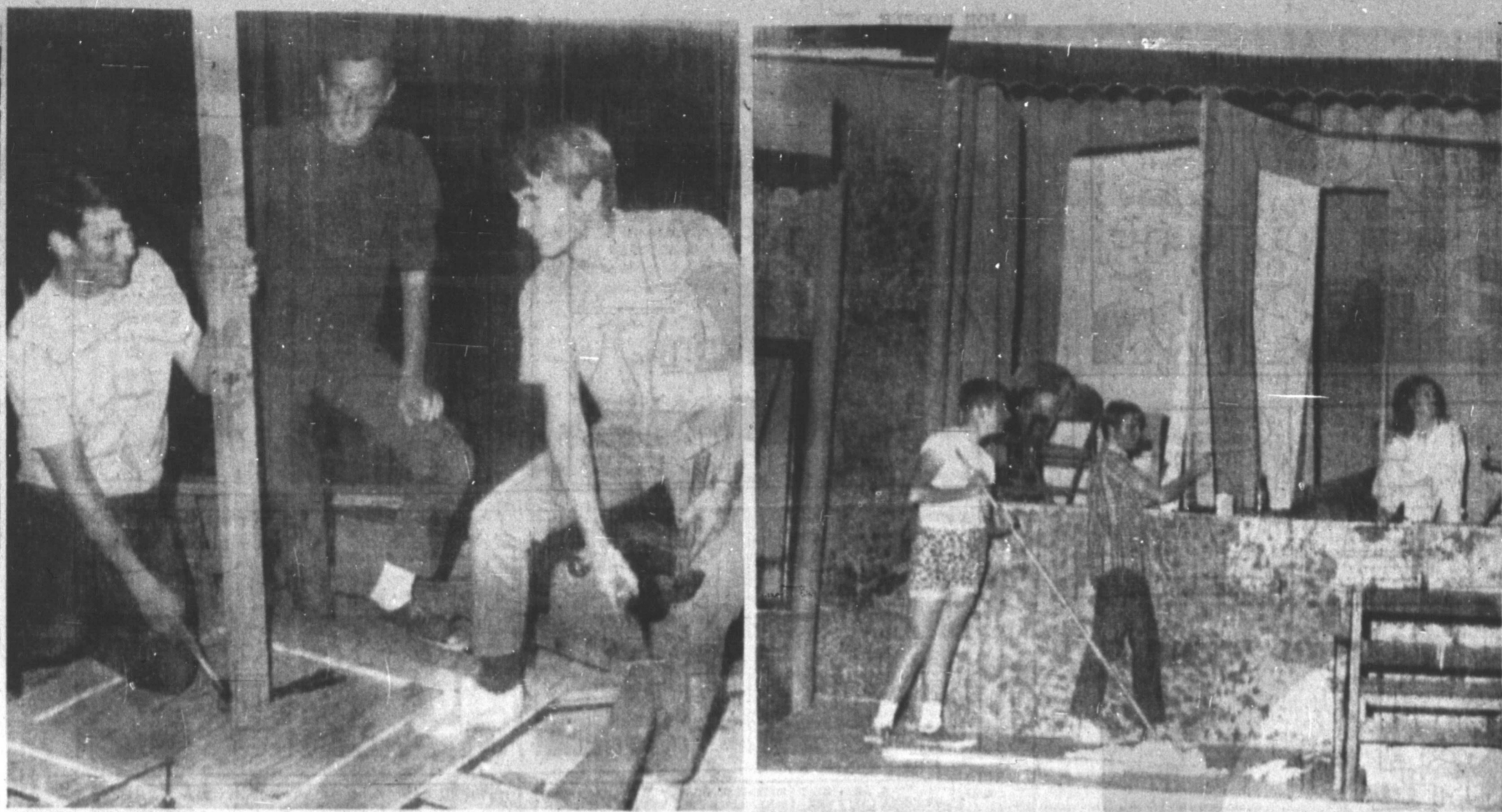
PICTURED ON the left Curt Morrison, Alnn Duck and Jeff Dunn as construction on the revolving stage was begun... on the right, the revolving stage is all most completed for Friday and Saturday night performances. (Staff Photo)
