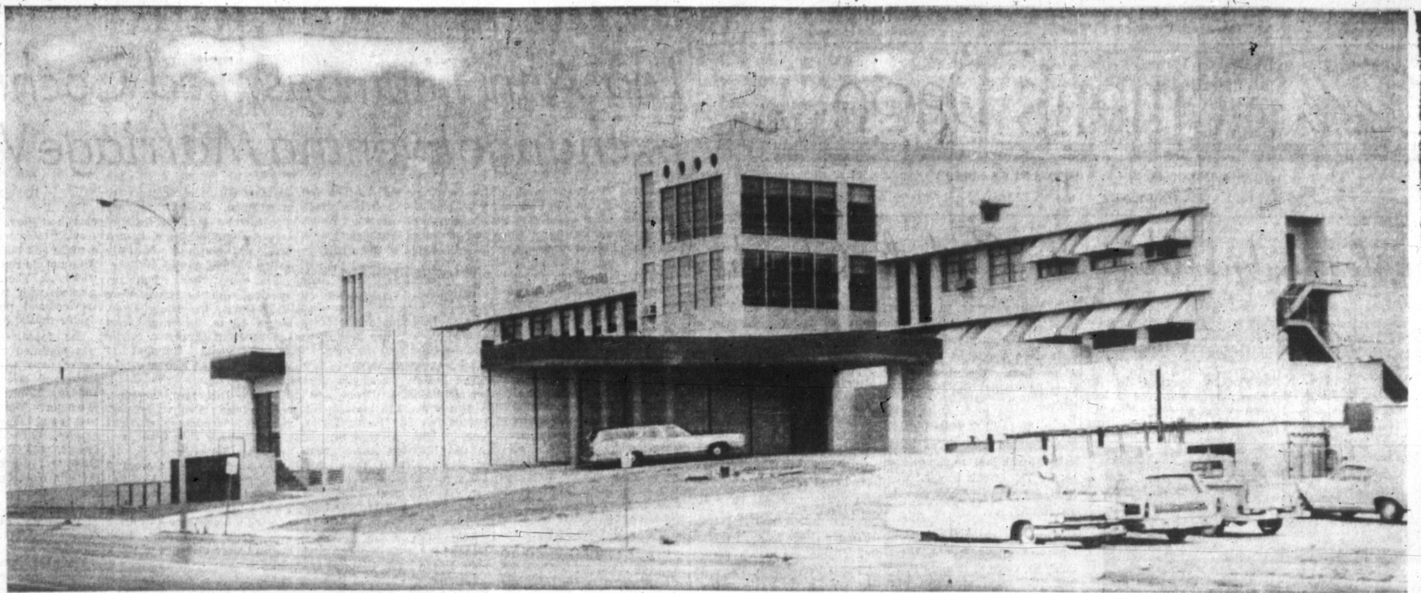
A NEW FACE on Highland General Hospital greets passers by on Hobart Street. An emergency drive-way, is just one of the new improvements made in the $1.4 million project. Completion date for all construction is Nov. 25. Bonds and federal funds have financed the construction project.
