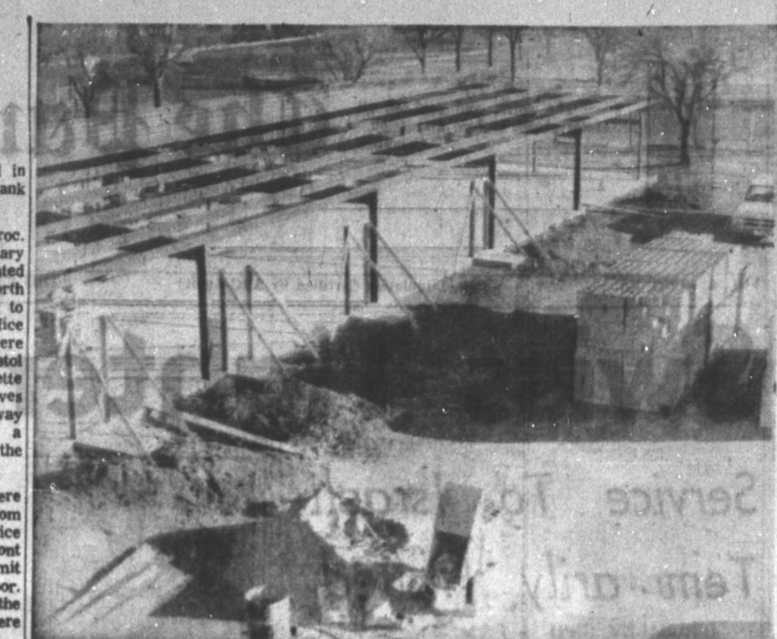
CONCRETE AND STEEL forms the framework for the $92,699 Pampa High School athletic field house constructed near PHS tennis courts. Hallmark Builders, Inc. have 50 per cent of their work, the plumbing, concrete foundation and steel wall frame finished and have until April 15 to complete the 21,000 sq. ft. steel building which will be used as an indoor workout area, with dressing rooms, offices and squad room for boys' athletics. (Staff Photo)
