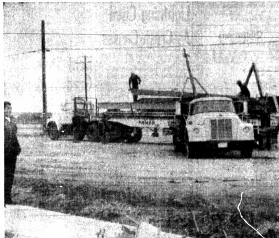
STEEL BEAMS to be used in the reconstruction of the county annex building east of the city are being unloaded at the construction site as Project 2 Commission 1 Vernon Walters left today on Reconstruction of the annex, destroyed by a tornado April 18, will begin as soon as debris clearance has been completed. (Staff Photo)
