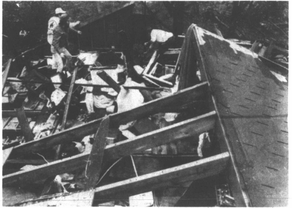
ROOF DESTRUCTION —A tornado which struck the Rogersville, Mo. area Tuesday hit the rural home of Paul Ewing, leaving half the
