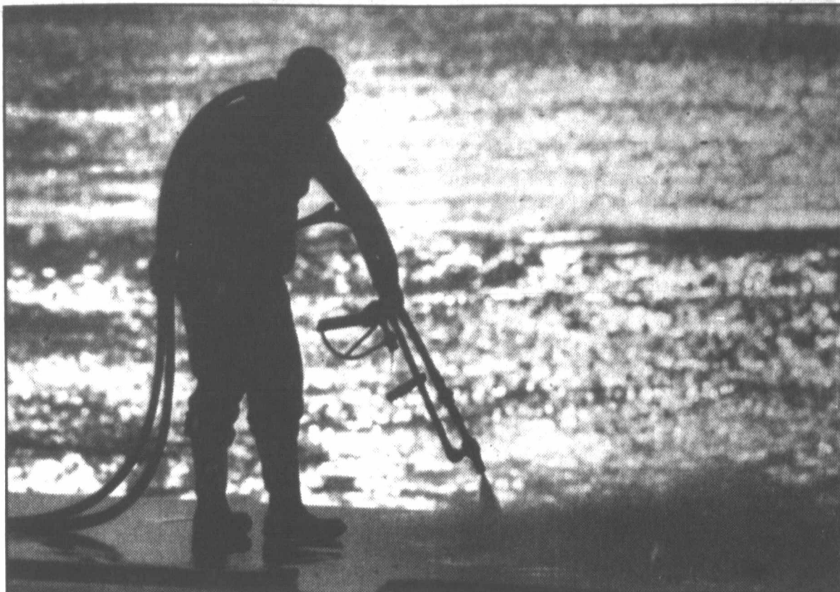
CLEANUP CONTINUES—Felix Orozco of Coastal Hydro-Vac Co. of Texas City cleans the Galveston Seawall using a hydro-blaster under 6,000 pounds of pressure to remove the tar deposited on the seawall in the recent oil spill. All that remains to be cleaned is the top of the seawall and the rocks at its base.
