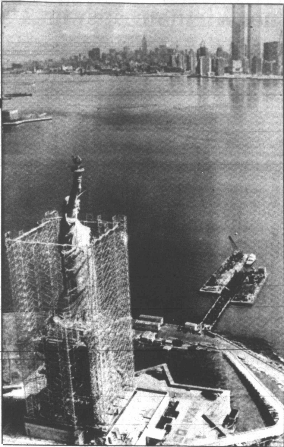
NEW LOOK FOR MISS LIBERTY —Scaffolding rises around the Statue of Liberty, forming a cage of pipes around the landmark and national symbol in New York Harbor. The scaffolding is the first step in a $30 million renovation project which will give the proud lady a new look for her centennial.
