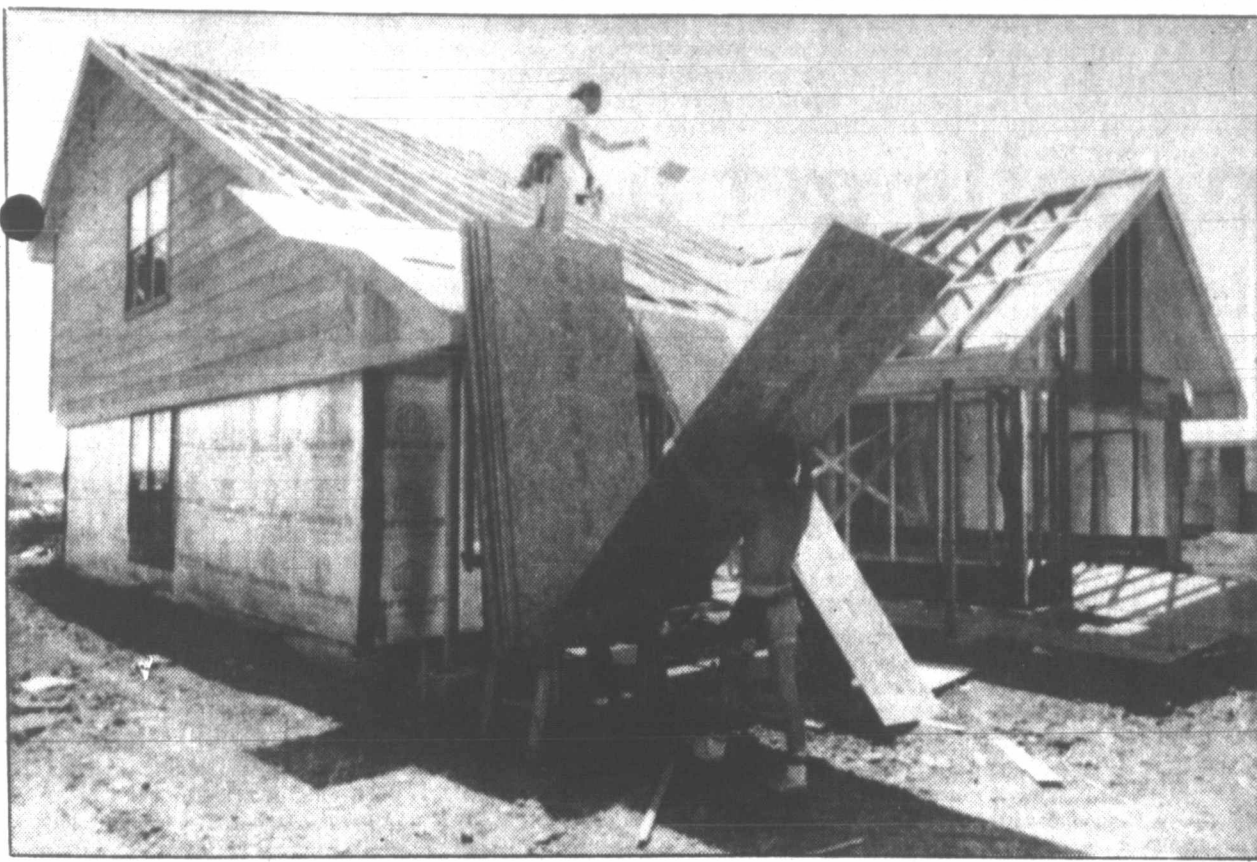
ON THE EDGE—Construction workers John Clement, below, and Jerry Fleming resume work on a Grand Prairie house which President Reagan chose to visit Thursday. Reagan told the workers they are out in front of the construction industry's comeback with the building boom that the Dallas - Fort Worth area is experiencing. (AP Laserphoto)
