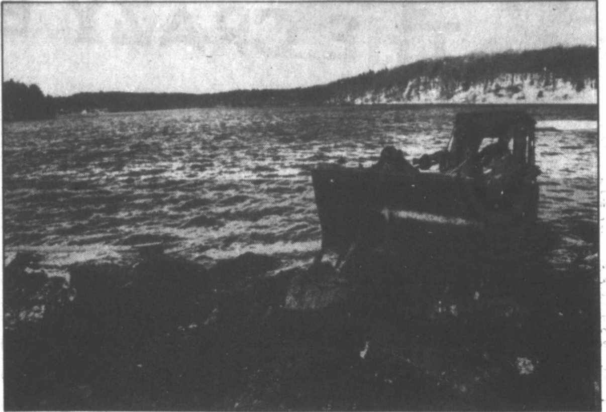
WALDEN RENOVATION—Man driving bulldozer clears debris from the beach at Walden Pond in Concord, Mass., recently as part of the effort to return the pond and the surrounding area to the condition it was in when philosopher Henry David Thoreau lived nearby.
