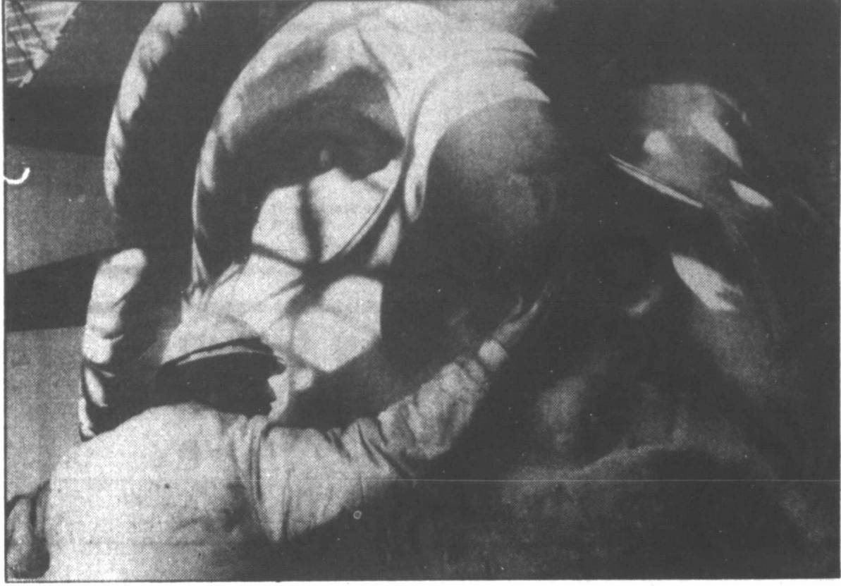
NOSE TO BE FIXED—Part of the serious damage to the nose of the Statue of Liberty gets a close check by safety engineer Angelo Joseph on Liberty Island in New York Harbor. The
