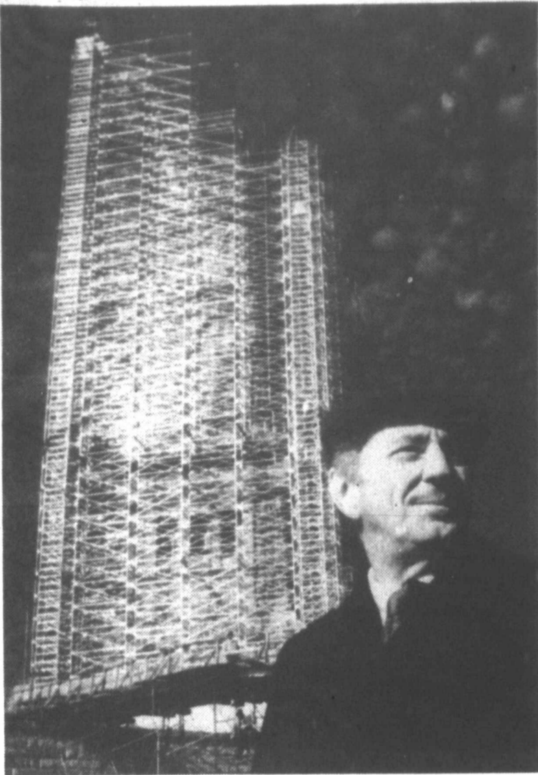
RESTORING THE BEAUTY —Larry Ballante, partner in an engineering, architectural and design company that is providing technical advice for restoration of the Statue of Liberty, approaches the statue covered with scaffolding, aboard a boat in New York recently. "The number one goal is to put her back in a physical condition that will allow her to survive the next 200 years," Ballante said of the restoration project. (AP Laserphoto)
