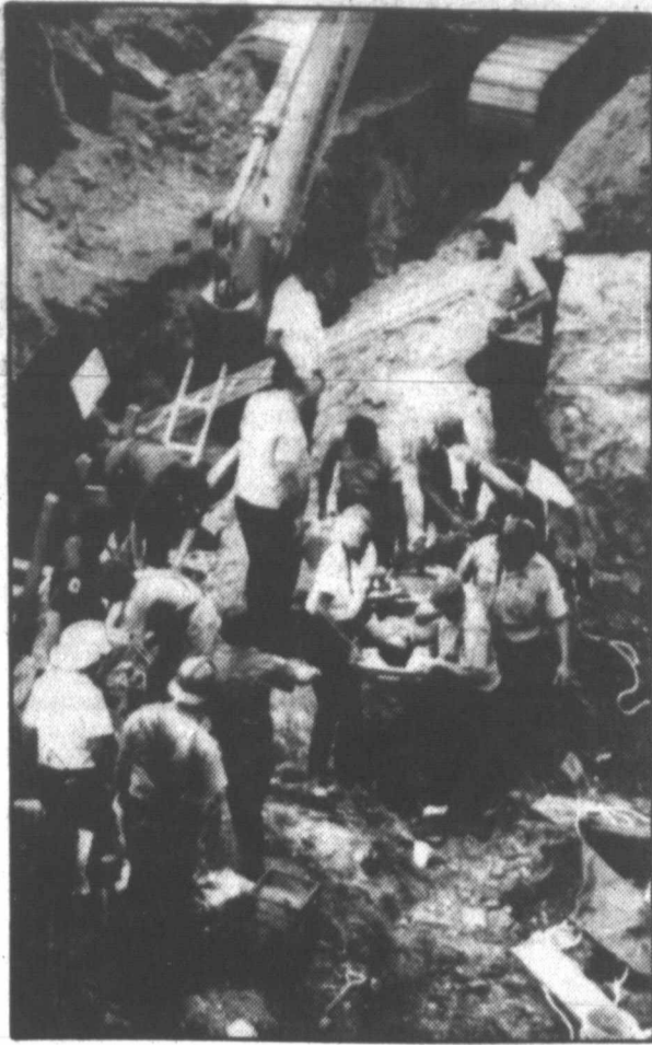
RESCUED FROM CAVE-IN —Rescuers carry 21-year-old Chuck Jones of Atlanta from a construction site where he was buried under tons of dirt and rocks for nearly four hours after the walls of a ditch caved in on him Monday afternoon. The construction worker suffered a broken leg in the ordeal. (AP Laserphoto)
