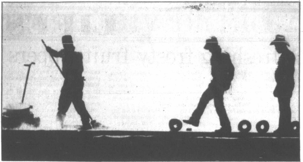
RELIGIOUS ROOFERS —Three men work on roofing the top of a San Angelo church Tuesday afternoon. One roofer is mopping down hot tar on the roof as another man rolls out the roofing paper over the tar. The third man followed by walking over the roofing paper to make sure it was secured to the tar. (AP Laserphoto)
