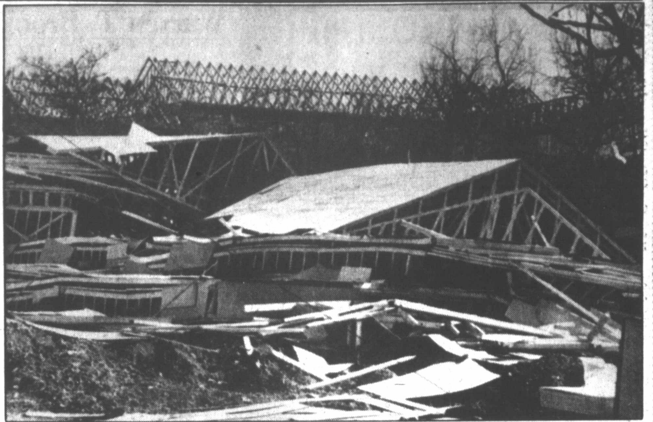
STORM DAMAGE —Part of an apartment complex under construction in San Antonio tumbled down due to high winds Sunday. The three-story structure was near completion until five tornadoes reportedly touched down in the San Antonio area. (AP Laserphoto)
