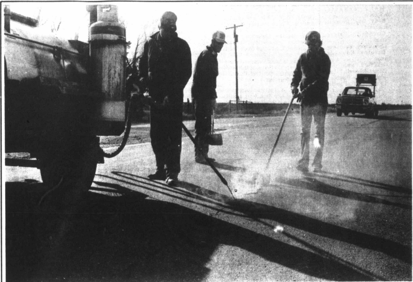
WINTER WORK —Winter's hardest blows have escaped the Pampa area so far, but employees of the Texas Department of Highways and Public Transportation know they'll hit eventually and they're getting area highways ready. This crew is sealing cracks along U.S. Highway 60 to prevent moisture from freezing and cracking the roads. This is a normal winter chore for the highway department and it will continue throughout the cold months. In this photo, from left, are Len Mixon, Wallace Fritz and Danny Smith. (Staff photo by Ed Copeland)
