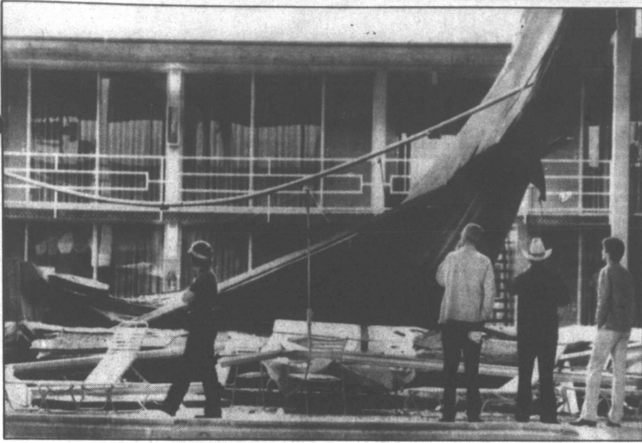
ROOF COLLAPSE — Police and spectators view the debris after a section of roof over a Holiday Inn Holiday pool and recreation area in Midwest City, Okla., collapsed. Officials said the roof collapsed Tuesday morning after a heavy downpour dumped more than an inch of rain in less than 30 minutes. No one was injured. (AP Laserphoto)
