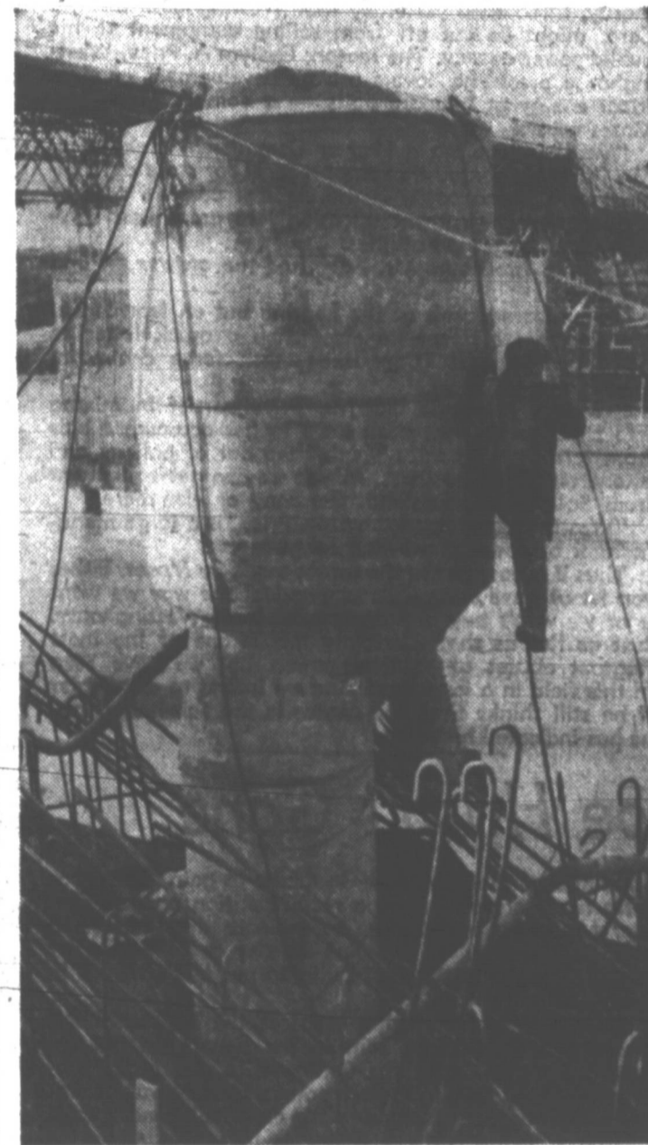
FOR DARK HOURS —A workman prepares to go under the Tiber River in Rome in a pressure tube to the foundations of a dam which will give the city electricity from a source right at its doorstep. In addition, the dam will furnish water for a vast cultivated area, boosting Italy's agriculture. The dam is due for completion some time next year.
