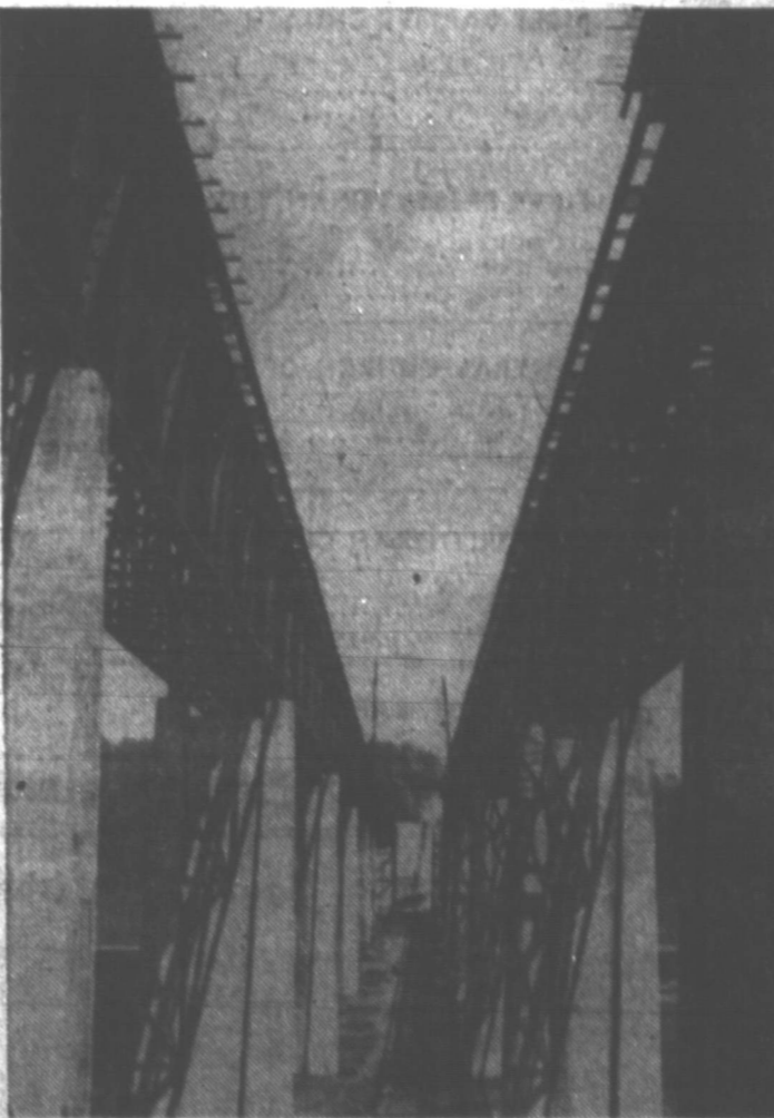
SOME TIME NEXT YEAR —Concrete, steel and sky make an interesting contrast as these two bridges are constructed over the Cuyahoga Valley at Peninsula, O. The twin spans are part of the new turnpike being built across Ohio. One end of the 241-mile stretch is connected to the Pennsylvania Turnpike, and the other ends in a pasture at the Indiana border. The $326,000,000 project is scheduled for completion on November 1, 1955.
