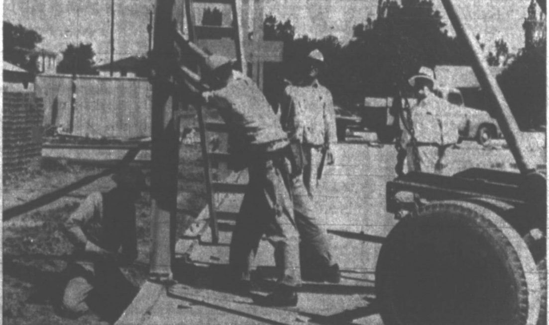
ERECTING LIBRARY STEEL — Lovett Memorial Library workers this morning were erecting the structural steel which arrived in Pampa last week. At the left is T. E. Kelly, Lubbock, who is putting in a bolt at earth level. Pushing up a steel beam are K. W. Trumble (in the foreground) and Bill Baker (behind him), both of Lubbock. All three are employed by Hardy Steel Erectors, Lubbock. Looking on in the background at right are C. E. Ratliff (left), White Deer, Tri-State Construction company job superintendent, and Albert Olson, 436 N. Carr, superintendent for E. E. Cantrell, local architect who designed the building on Houston, between Foster and Kingsmill. (News Photo)
