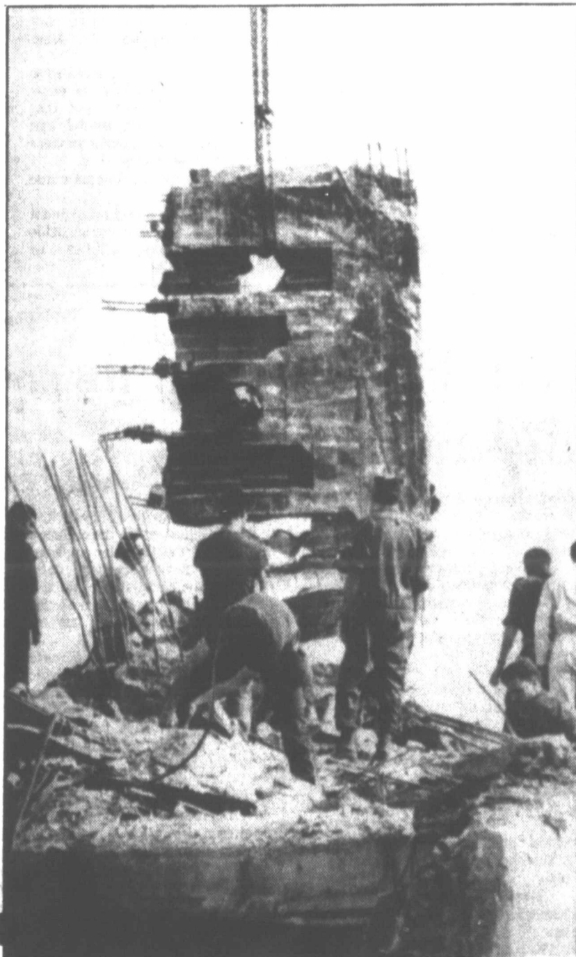
DIGGING CONTINUES—U.S. Marines, aided by Lebanese rescue workers and Italian troops of the multinational peacekeeping force, continued to lift slabs of concrete in
