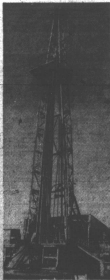
LET 'ER BLOW —The wide open spaces of western America aren't the only areas where "black gold" fever runs high. This towering oil derrick has risen in Exmouth Gulf, Western Australia. Pipes rise from the ground inside the derrick as the bit descends into the earth and diesel engines begin to pulse near the base of the structure.
