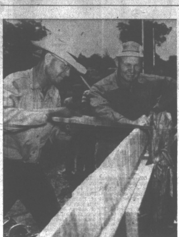
PUTTING ON FINISHING TOUCHES — Shown above are two of the many Pampa men who have helped in building the Little League and Pony League parks. With saw is Bill Ridgway, manager of the Cabot team in the Eastern Little League. At right is R. L. Chase. The two are shown putting the finishing touches on the fence at the Eastern Little League Park located on the Lions Club Park grounds. The other two kid parks are located just east of Fisher Granary. Local citizens are invited to be on hand for the season opens tomorrow in all three leagues. (News Photo)
