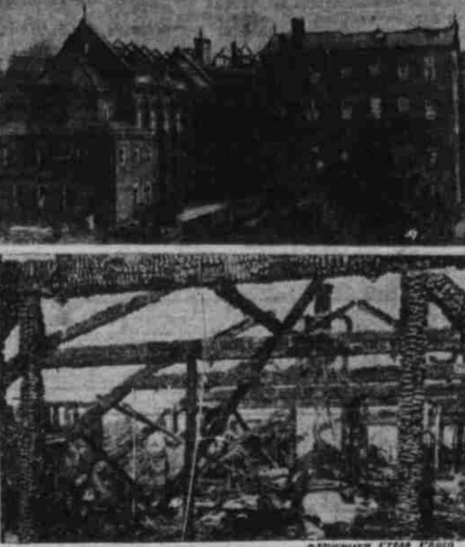
The Little Sisters of the Poor Home for the Aged in Pittsburgh, Pa., after it had been swept by a fire which resulted in 40 deaths. More than 200 were injured. Lower picture shows the ruins of the third floor where many of the inmates perished.
