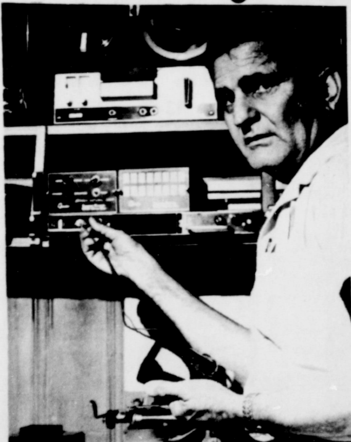
Jim Crabtree, of the DACO Company, Dallas, is shown making final adjustments on Quindar Telemetering Receiver-Scanner recently installed at A-1 Answering Service, Eastland. Unit monitors vital functions of new Odessa Natural Corporation's Carbon Compressor station, 24 hrs. per day.
