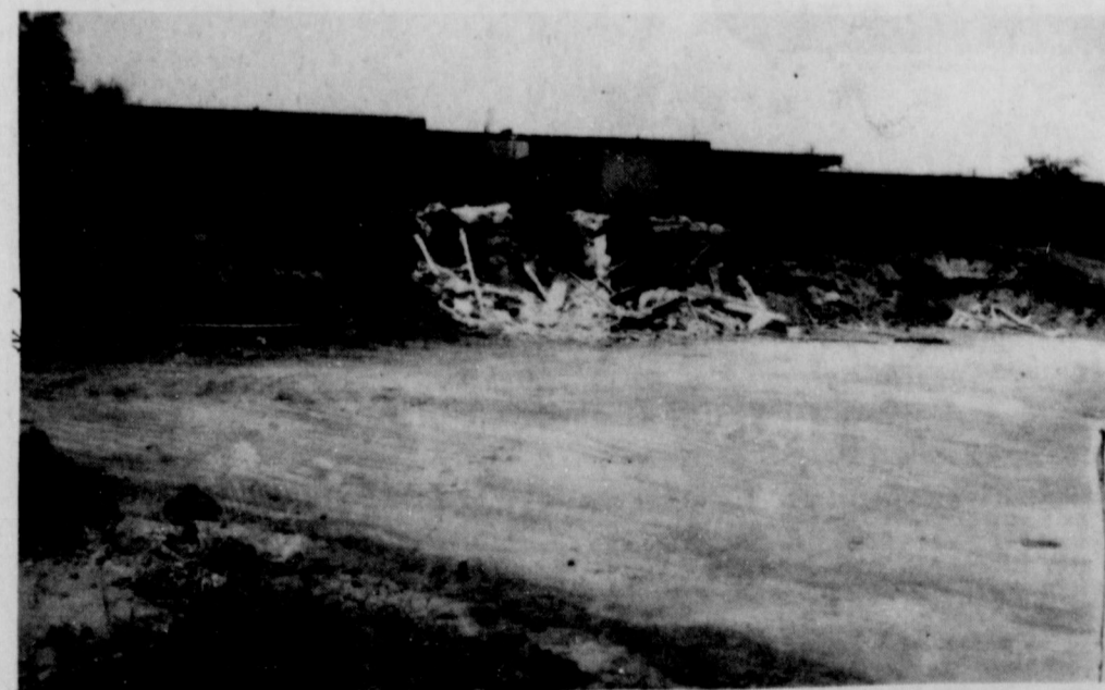
Construction is underway on the new Hospital expansion program. Pictured above is the east side of the hospital with the ground already smoothed off and part of the hospital under construction.
