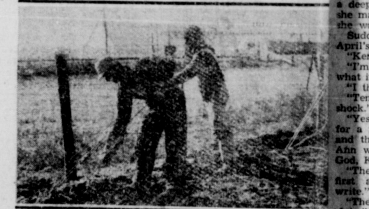
One reason why the giant poles of electric distribution and transmission can withstand the terrific strains that they do is because they are securely wherever possible. Here Haskell Wadkins and Wayne Gregston of Midland secure the guy wires on a transmission line dead-end.
