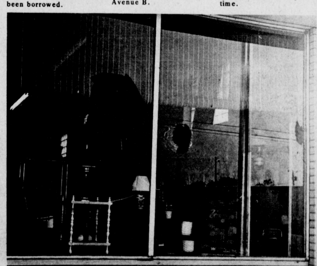
A TRAIL OF BROKEN WINDOWS --Gunn Brothers Stamp Redemption Center, shown here, is one of six businesses vandalized by rock throwing individuals during the night Thursday. Three rocks were thrown through the display windows shown here. The large hole at the left, a smaller one in the center windows and another of the same size in the window at the far right. Also losing windows were the post office, Bailey County Electric Cooperative, Muleshoe Electric, Lindsey Jewelry and the Merle Norman Studio.
