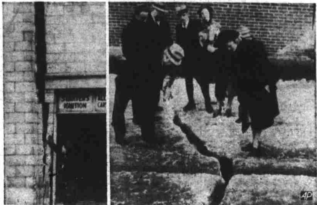
BUILDINGS SPLIT, STREETS CRACK AS TOWN SETTLES—Slowly widening cracks split the walls of homes and business places (left) in Shetandeah, Pa., where the town's most heavily populated section settled as much as 20 inches due to mine cave-ins.
