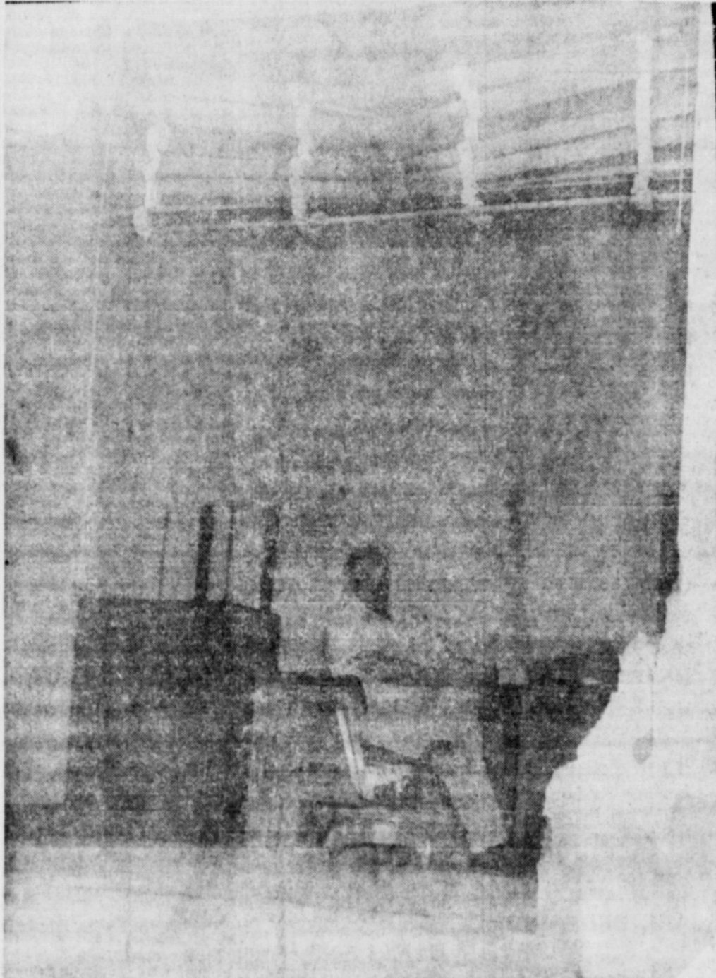
UN-INTENDED VENTILATION — Joe Manning, Foremost Distributor, sits at his desk and looks out through what was the east wall of the building. An auto collision about a block away Friday morning caused the damage when one of the vehicles crashed into the building, causing considerable damage, but injuring no one in the building. Marlin Cagle was injured in the crash.
