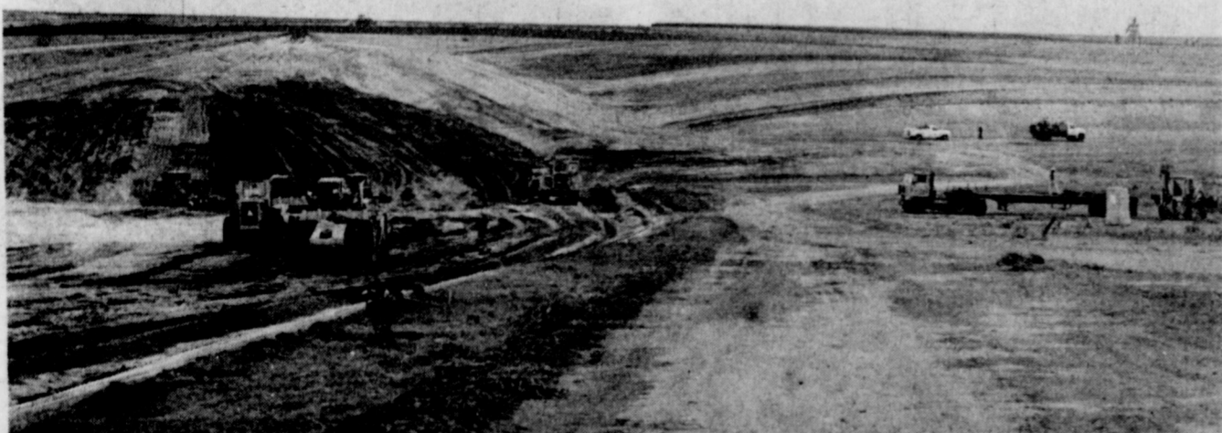
NEW DAM SITE...The lake shown above, located approximately five miles northeast of Lazbuddie, will contain 453 service acres of permanent water. The dam will be 51 feet high at the tallest section and the deepest spot to the dam will be 27 feet. The dam is 12 percent complete and will be finished in approximately one year and
