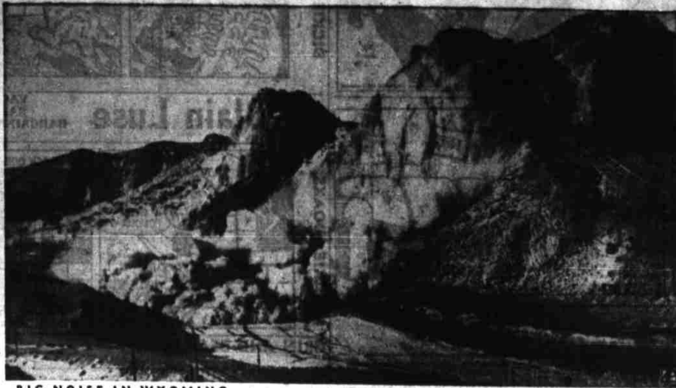
BIG NOISE IN WYOMING —Contractors on the Geyser Dam, Wyoming, needed 150,000 cubic yards of rock fill so they exploded two carloads of TNT in the side of a mountain along the Wind River. The roar could be heard fifty miles away.
