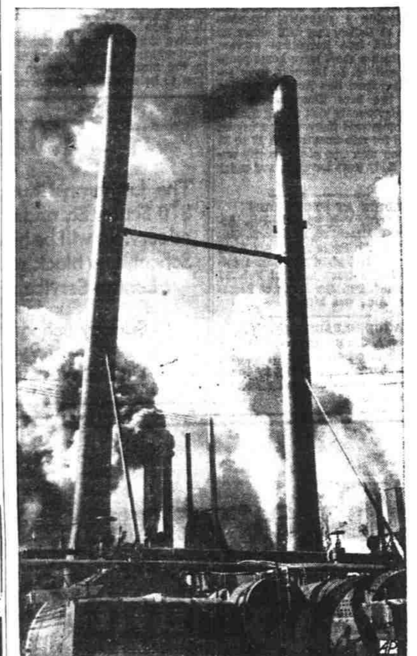
PACIFIC PITTSBURGH —Smoke billows from stacks in a forward area war plant deep in the Marianas, within bombing distance of Japan. It's an asphalt-mix plant set up by aviation engineers in the jungle.
