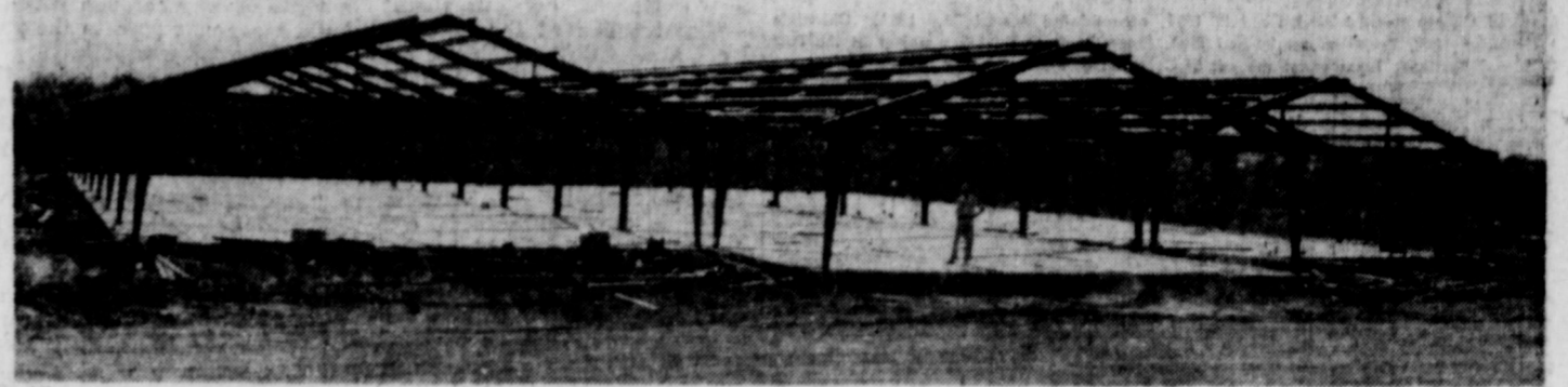
IT'S GOING UP—The new home of the Hollywood-Maxwell Corset Co. is going up fast and completion of the building is expected by Sept. 15, the contractor said this week. Framework of the building is pictured above. Actually work is even further along now than the picture reveals. (Canaris Photo).
