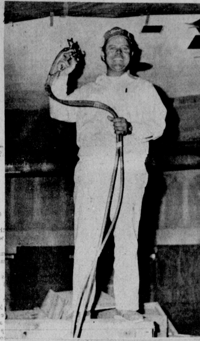
CEILING WORK... Although the weather has turned bad outside, work continues on the interior of the new First National Bank building. A workman here is installing a ceiling in a portion of the bank.
