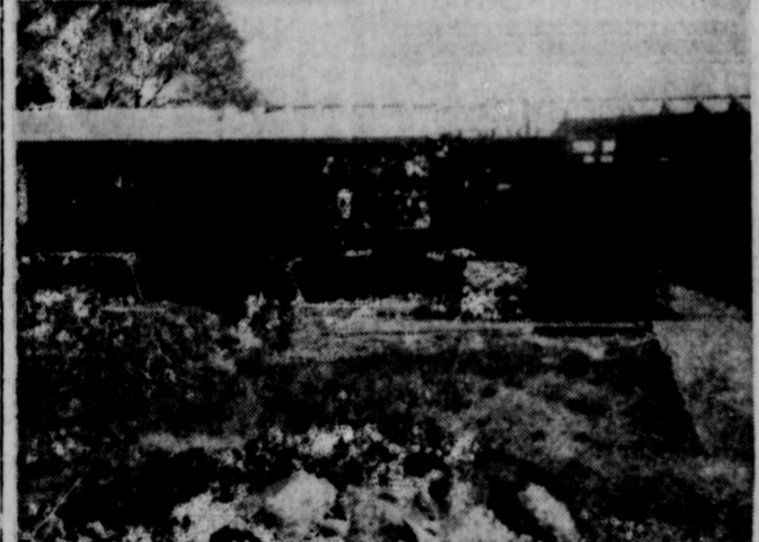
CONSTRUCTION UNDER WAY on this second Broyles-Built home, located on E. Lens St., on a site purchased from the school, on what was formerly Southward School property.
