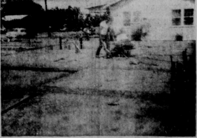
FOUNDATION preparation is underway and will probably be poured Tuesday for the Buck Wheat-built house in the 700 block of S. Sadosa St. This is the first of three to be built on this street by this party.
