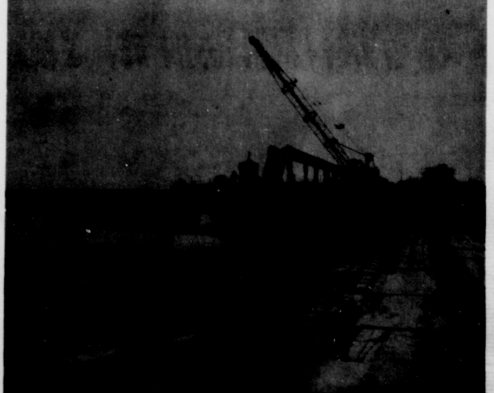
MAKING WAY FOR THE NEW - Progress is well underway on the new bridge that will span the Lake Eastland Channel northwest of town as the old bridge at right continues to serve. The expansive development is part of the new farm to market road development which will eventually link Highway 80 to 183, north, at the Y. Photos by H.D. Alsup
