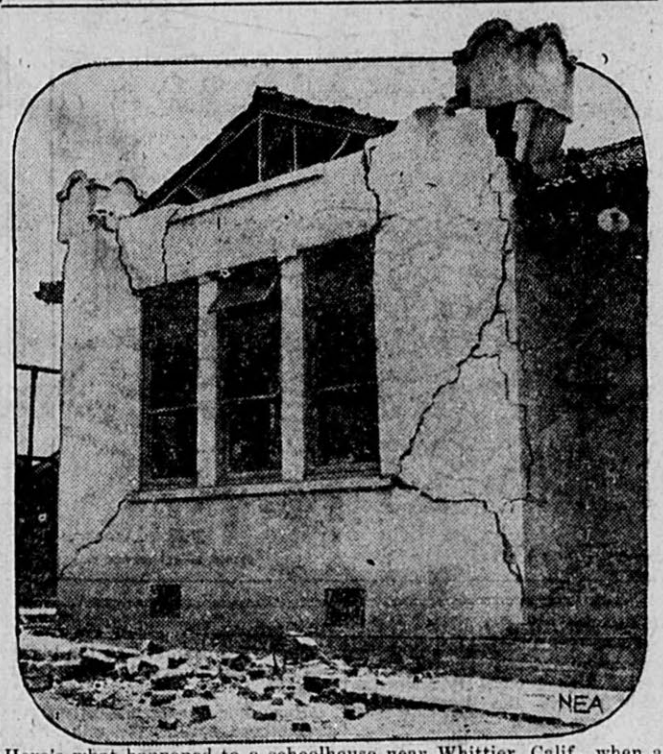
Here's what happened to a schoolhouse near Whittier, Calif., when a slight earthquake jolted the southern portion of the state the other day. No serious damage was done, but cracked walls, broken windows and loosened roofs gave citizens a number of thrills.
