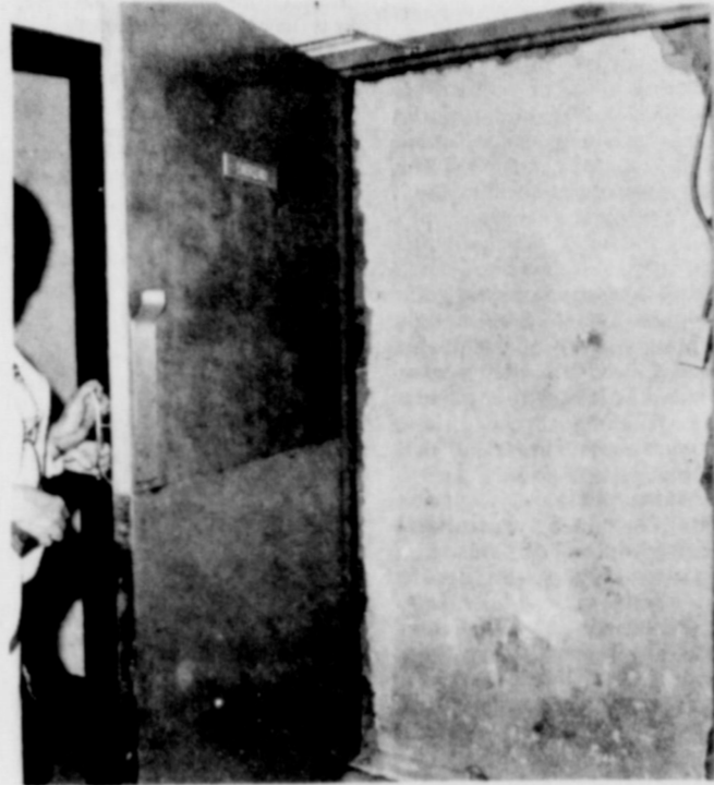
A person might think that a practical joker is lurking around the new portion of the hospital, but this is not the case. The wall is what is left of one of the old wings of the hospital and will be knocked out as soon as the newly completed emergency and other adjoining facilities can handle patients. (Photo by Steve Haines.
