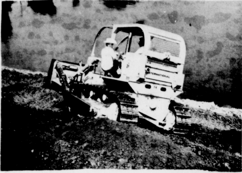
Operating his bulldozer in a very precarious position is Lindle Garrett, of Eastland. Lindle works for Bob Carroll construction, and are presently making a 2000 yard fill across a 110 foot section of its Lake Leon Dam. A portion of the dam eroded during the heavy rains this year, carrying part of the highway and embankment hazards to motorists, as well as to the stability of the dam. (Photo by Steve Haines).
