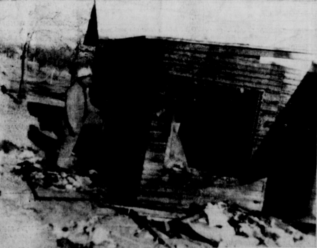
INSPECTING FIRE DAMAGE — Fire Chief Guy Robinson inspects damage to a room and its contents of clothes at a North Oaklawn home Friday afternoon. Fire is believed to have begun in this room, destroying much of the belongings of Mrs. Zerena Stull of 214 N. Oaklawn. Clothing belonging to Mrs. Stull and her five children was destroyed in the fire which began about 4:30 p. m. Firemen put out the blaze, saving damage to the rest of the house. The home is owned by C. N. Lindley. Mrs. Stull works as a waitress and her children range in age from two to eleven years. The woman was slightly burned about the head and face, was treated and worked Friday night at her job. The children were not injured, it was reported. (Staff Photo).
