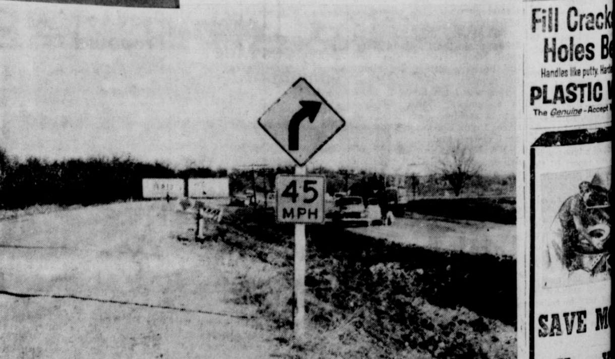
NEW CURVE —The $533,283 Highway 6 job now in progress includes the virtual elimination of the sharp right turn (old highway shown at left) as it nears Eastland. Right-of-way is already cut and dumpsters, seen on the new roadway at right, are now in the process of filling the roadbed. The road will veer eastward into Eastland with less curve, making for safer driving. Quite a few automobiles have failed to make the curve over the past years, and many have come to rest at the foot of the billboards which stand at the point of the curve. (A&C Photos)
