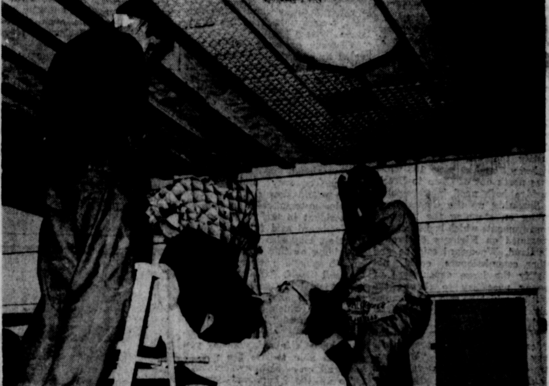
EGG CARTON EXPERTS —Four members of the Band Boosters Club are shown putting the egg carton fillers in place on the ceiling of the main rehearsal room of the new band hall. The fillers were used for acoustical effect. From left to right are Ray Pryor, Phillip Hewett, Wayne Jackson and Marlin Cagle. (Canaris Studio Photo).
