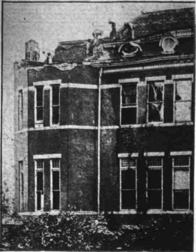
A local tornado caused about $10,000 damage when it hit Columbia, Mo., and swept a turret off Swallow hall, University of Missouri geology building. Workmen are shown repairing the roof.
