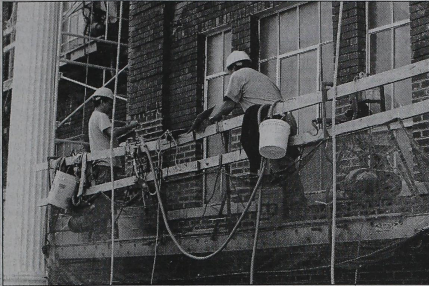
Mid Continent workers are busy replacing the mortar on the exterior of the courthouse. —Photo by Rob Schaffer
